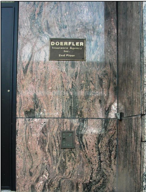
Figure 6. Cladding of the 3.5 Byo Morton Gneiss ("Rainbow Granite") on the exterior of an otherwise undistinguished bank building on Ridge Road in the historic southern suburb of Homewood. Some effort was made here to mount the panels so that the wavy foliation of this ancient metamorphic rock was oriented more or less vertically. (Photo by author)
